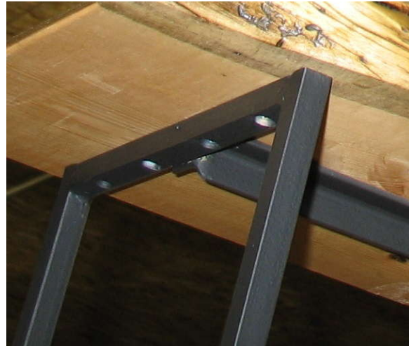
View of the underside of the top slab mounted to the cage.
